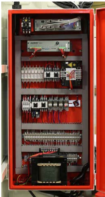
EVS-760B ELECTRICAL CABINET
